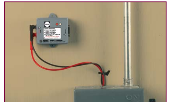
Model L215 monitoring a control panel looking for dropouts and spikes in the line voltage
