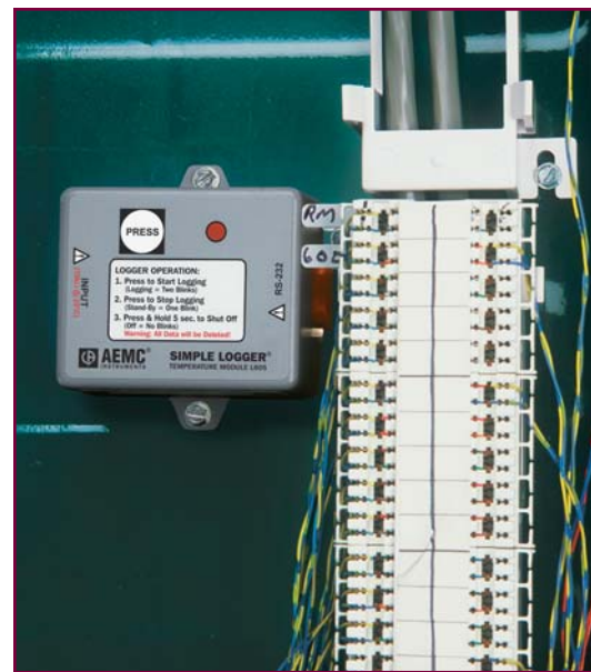
Model L605 monitoring the temperature in a communications cabinet
